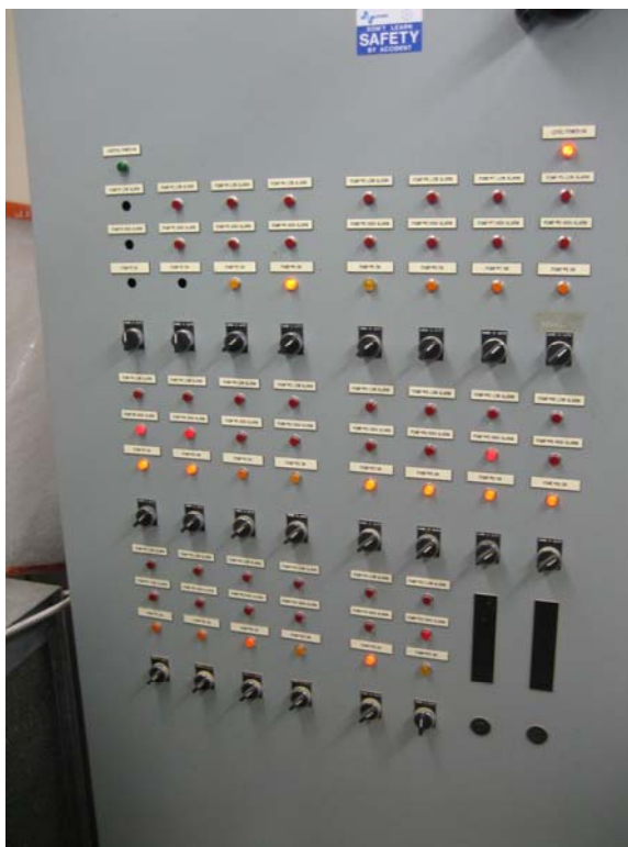
Control panel after system restoration (Site Visit -1)
