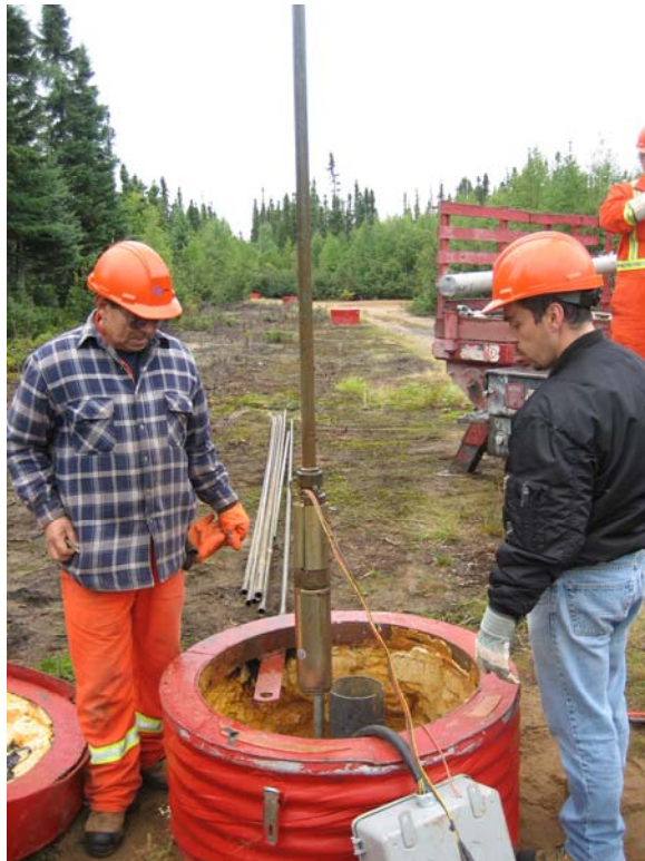
Pull-out of the pump in W4 (Site Visit -1)
