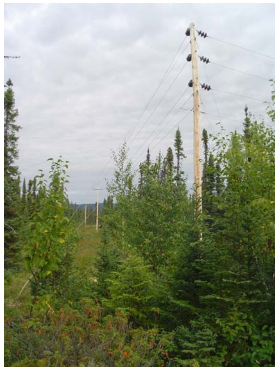
25kV Power to Control Shelter (Site Visit -1)
