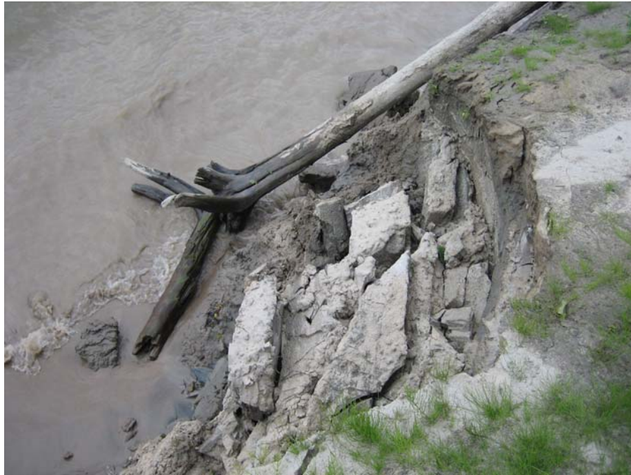
Erosion at downstream slope toe (Site Visit -1)
