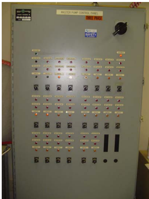
Common pump operation before the replacement of pump at W4 (Site Visit -1)
