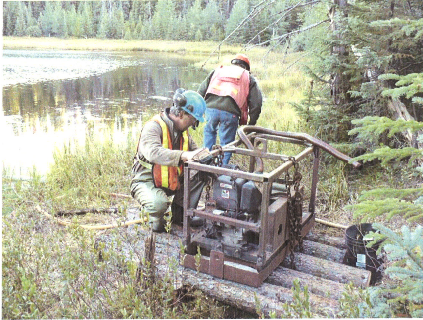
Photo 1 Water Supply Pump
