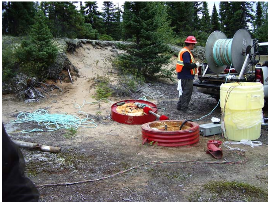
Photograph 8: An acid solution was added to the well and allowed to stand for 2 hours. Then a wellbore brush was used to clean the casing and screen.
