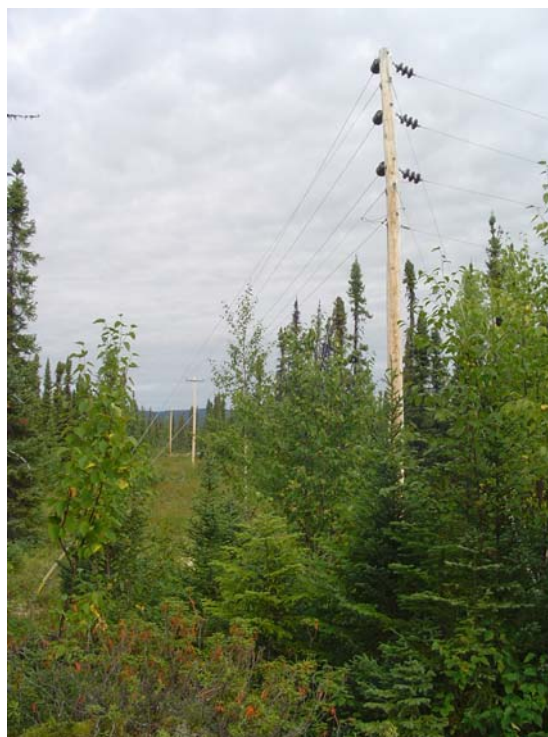
25kV Power to Control Shelter (Site Visit -1)
