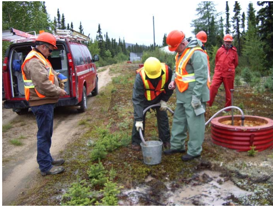
Photograph 1: A flow test was conducted at each well prior to inspection and cleaning.
