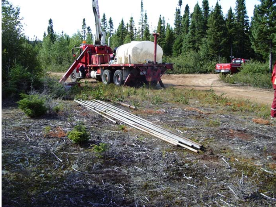
Photograph 3: The risers and pump were laid down on the ground for inspection.
