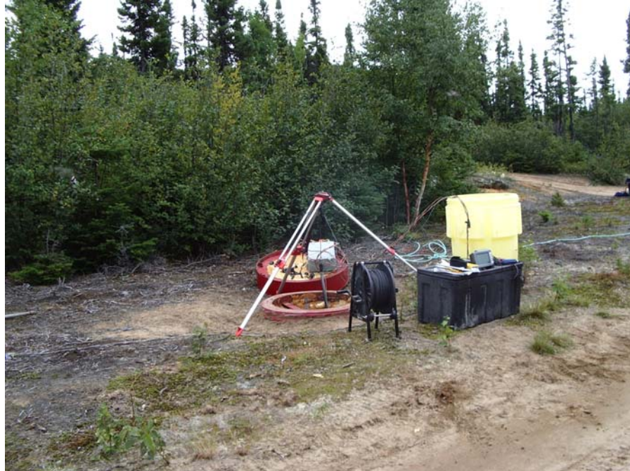
Photograph 7: A downhole camera inspection was completed before and after cleaning and logs made of the observations. The inspections were recorded as digital videos.
