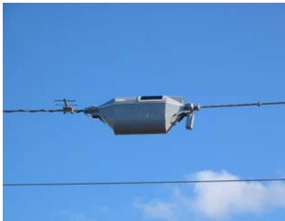
Fig. 18 Automatic ice control device installed on a 230kV line near St. John's
