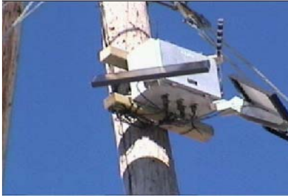
Fig. 16 CAT1 system installed on a 230 kV dead end structure
