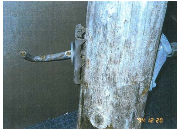
Fig. 4 Failure of a forged eye bolt in 1994
