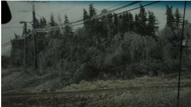
Fig. 21 Photograph showing the icing on distribution cable
