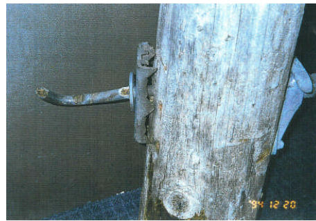
Figure 6. Failure of a forged eyebolt on a Wood Pole Dead End Structure - 1994
